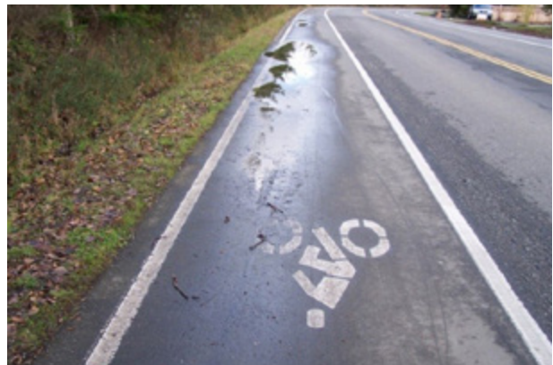
Figure 10.13 – Poor Drainage Causing Ponding in Bike Lane
