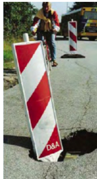
Figure 10.10 – Pothole Identified by Hazard Marker
