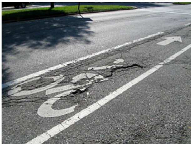
Figure 10.5 – Poorly Maintained Bicycle Lane
