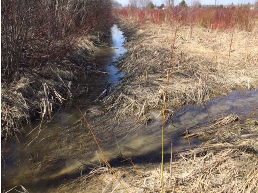
Photo 6. View of convergence of ditch flow on Galloway lands up-gradient of culvert conveying flow to Orsi lands (April 27, 2018)
