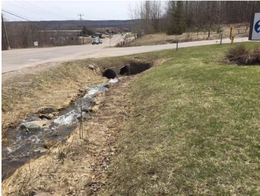
Photo 10a. Downstream view of flow within west ditch of William St at double culverts conveying flow under William St. to the east (April 27, 2018)
