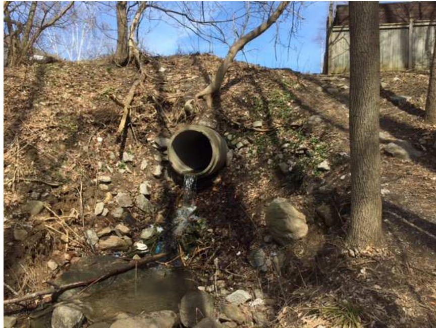
Photo 3. Discharge culvert south of Christine Dr. and Maxwell Ave. intersection that discharges to Galloway lands (April 27, 2018)
