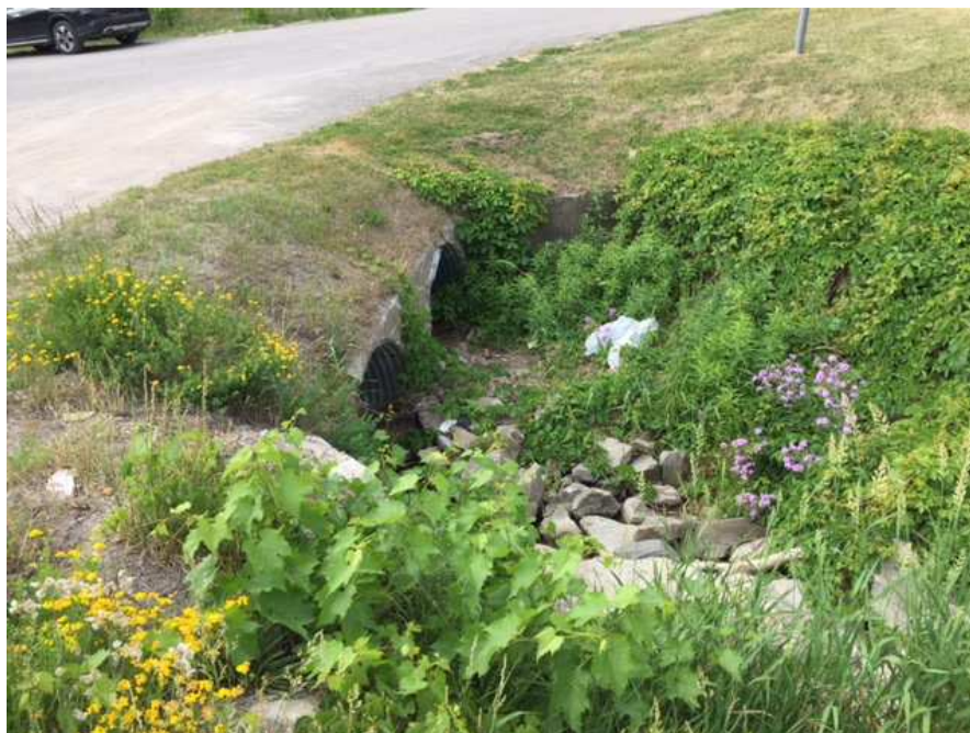
Photo 10b. Downstream view west ditch of William St at double culverts (June 13, 2018)
